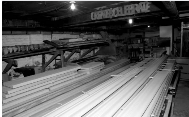
AFRICAN MAHOGANY TRIM WAITING TO BE INSTALLED AS PART OF THE EXTERIOR RENOVATION PROJECT. THE WOOD WAS CHOSEN BECAUSE, UNLIKE MAHOGANY FROM SOUTH AMERICAN RAINFORESTS, IT IS A RENEWABLE RESOURCE.
